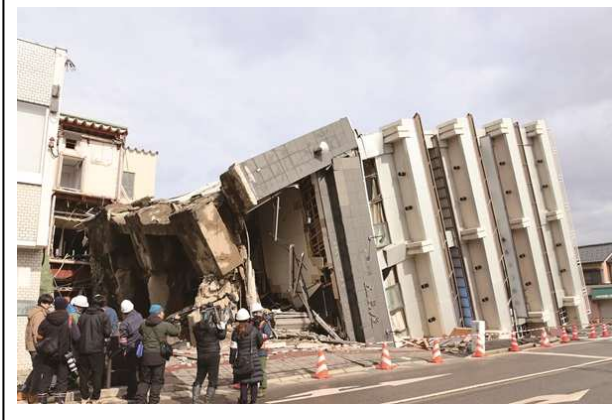
Photo 4 Kawai-machi, Wajima-shi – one of the towns struck by the disaster (Top: location of widespread fire, Bottom: collapsed building)
