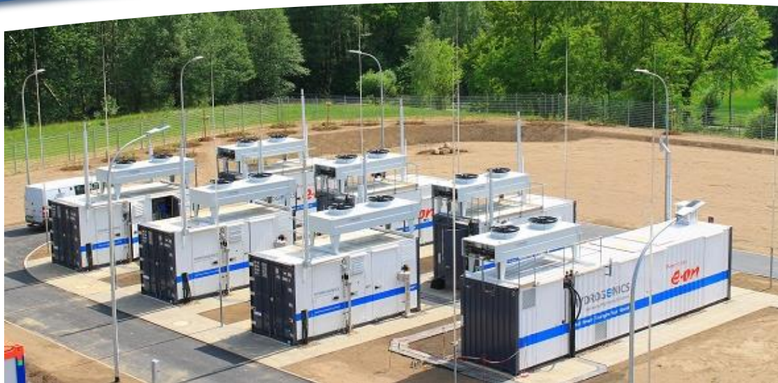
Power-to-Gas plant in Falkenhagen, Germany
